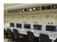
Plant monitoring and control system
