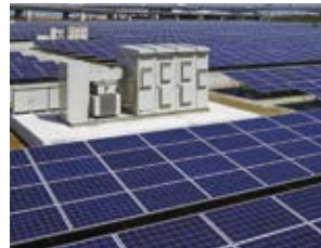
Solar power generation systems
