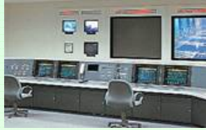
Plant control systems
