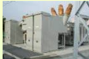
Power receiving and distribution substation equipment
