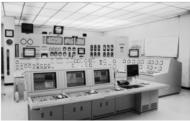
Fig.10 Central operation room, after renewal
