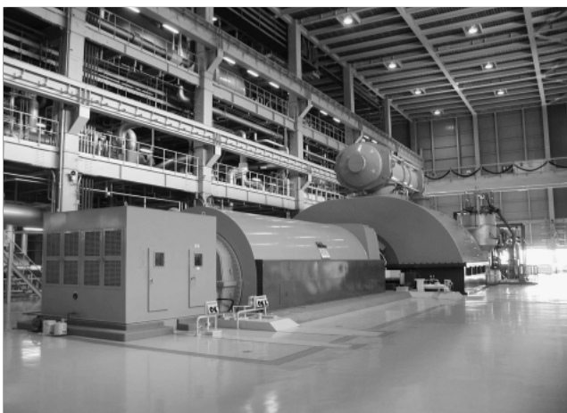
Fig.1 EPDC Isogo Thermal Power Station new Unit No. 1
