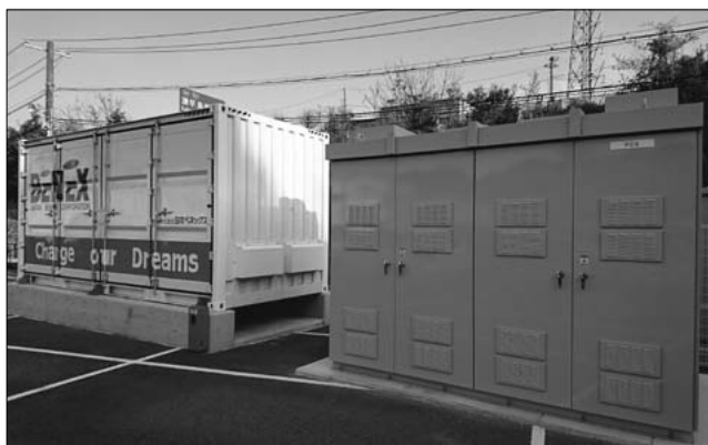
Fig.1 Used EV storage battery system
