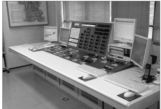
Fig.1 Dam monitoring console
