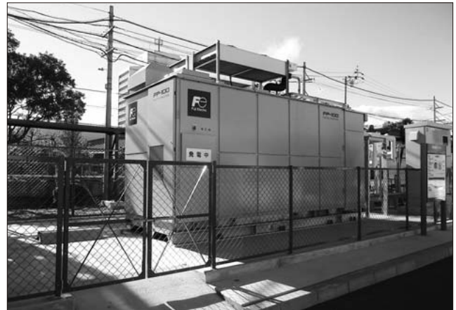
Fig.8 Fuel cell installed at Mie factory
