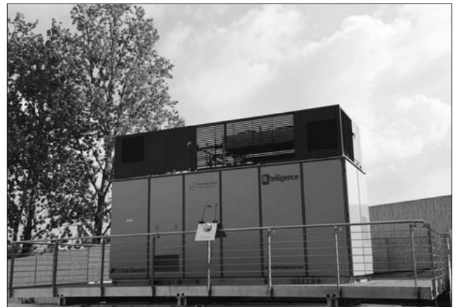
Fig.9 CE-marked fuel cell delivered to Germany
