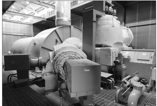
Fig.1 100 MW steam turbine and generator
