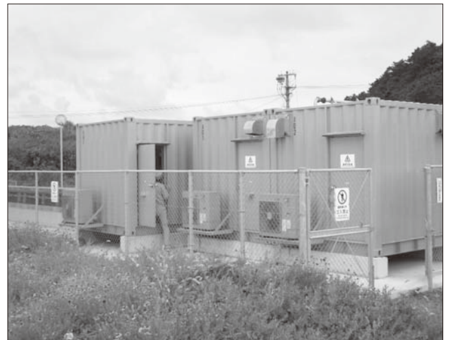
Fig.7 Appearance of storage containers
