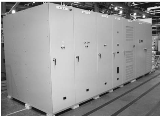
Fig.8 Overview of the 6.6 kV-2,000 kVA UPS (8,000H)
