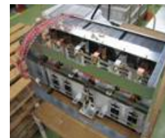
Power conversion unit
