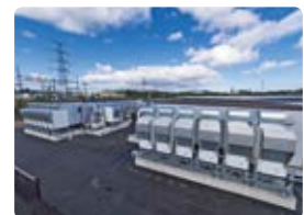
Data center using snow ice storage type cooling device
