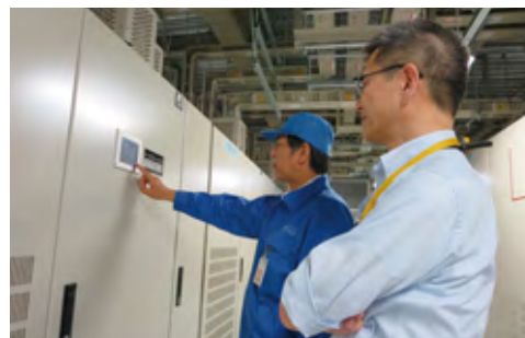
Inspecting a UPS unit
