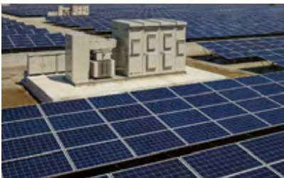
Kisozaki reclaimed land mega-solar
