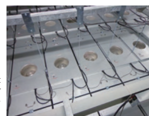
The Fuji Electric Fan Filter Unit with Inverter (clean room upper chamber) controls airflow optimally for each work area
