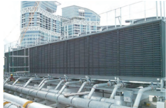
External unit of the air conditioner system installed on an office building roof
