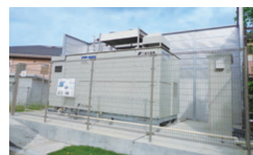
Fuel cells installed adjacent to a residential area
