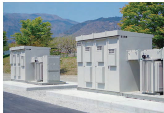
Fuji Electric power conditioners (1 MW x 2)
