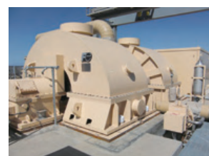
The turbine Fuji Electric supplied for HRI
