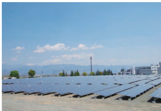
Solar panels installed onsite at the Yamanashi Factory
