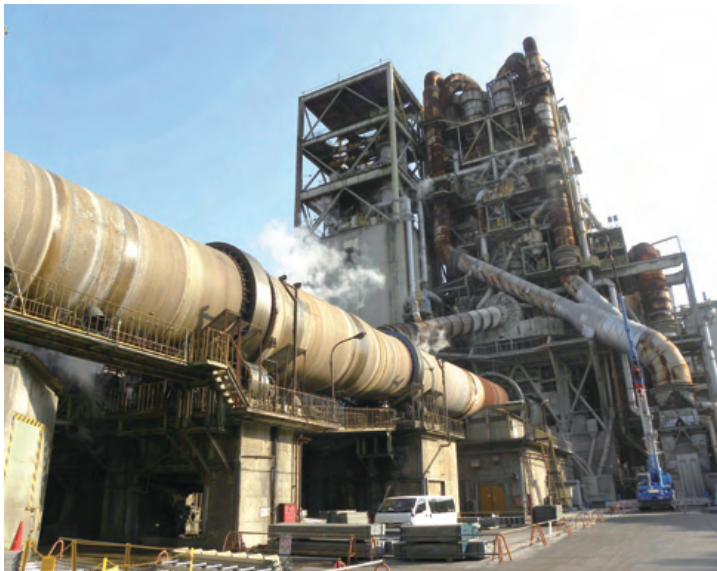
The cylinder in the foreground at the Saitama Plant of Taiheiyo Cement Corporation is a cement incineration kiln
