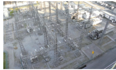
Power receiving and distribution substation equipment
