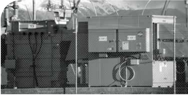
Example of a 4 MVAR D-VAR system, which is 20 feet long by 11 feet wide. D-VAR systems are modular and compact and accommodate areas with restricted space availability.
